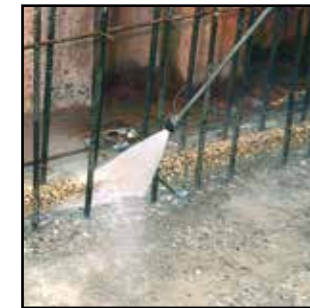
For improving the rough- ness of the work joint as well as the adherence with the fresh concrete, the work joint should be treated with a high pressure water gun.
