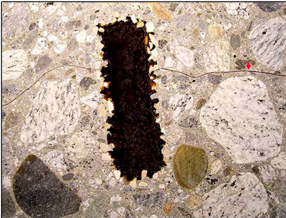
fissure in a concrete work joint
